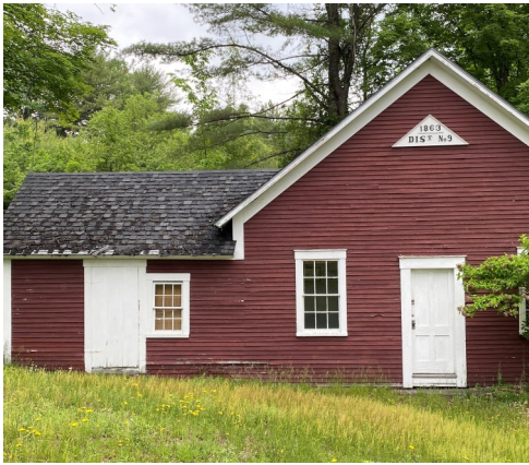
New roof and site grading are among planned repairs.
