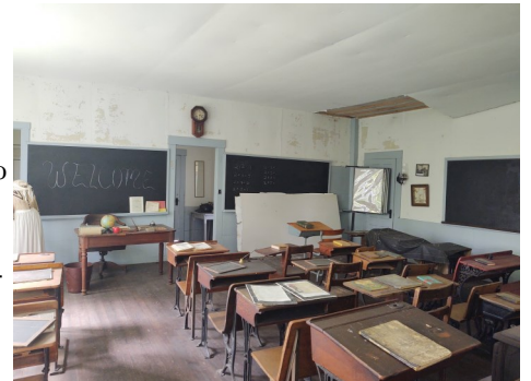
Schoolroom in need of repairs and paint.
